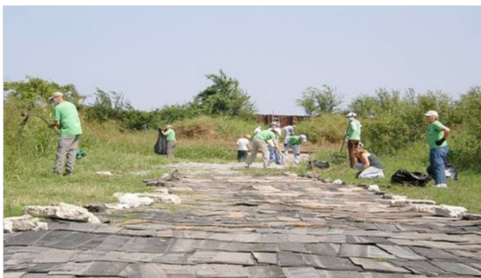
Figure 9: Volunteers clearing vegetation and establishing access to the sheet piling before the platform construction. (Photo courtesy of Daryl Malek-Wiley, 2007.)
