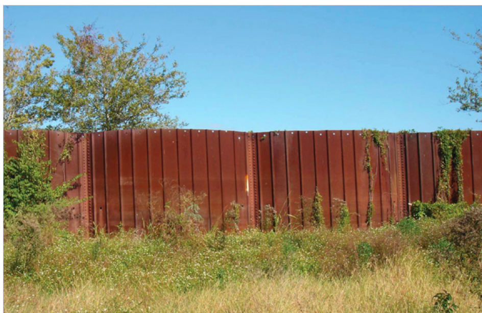
Figure 4: Levee and sheet piling along Florida Avenue, Lower Ninth Ward, New Orleans, 2006.
