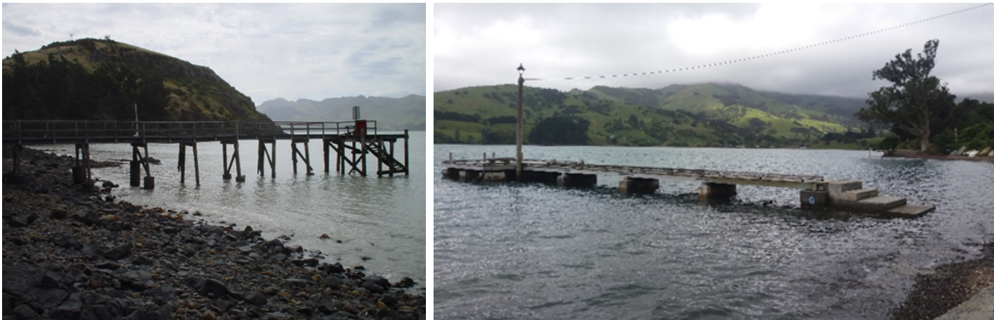
Figure 1 (Left): Kaioruru/Church Bay jetty 2007 – piles show degradation.
