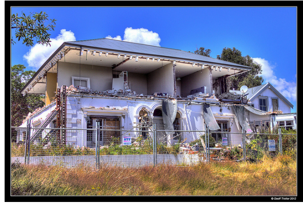
Figure 1: Godley House, post-earthquake (Geoff Trotter)
