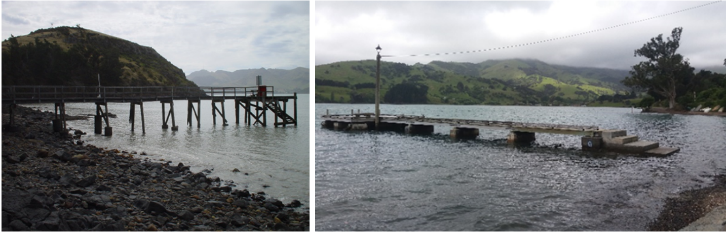
Figure 1 (Left): Kaioruru/Church Bay jetty 2007 – piles show degradation.
